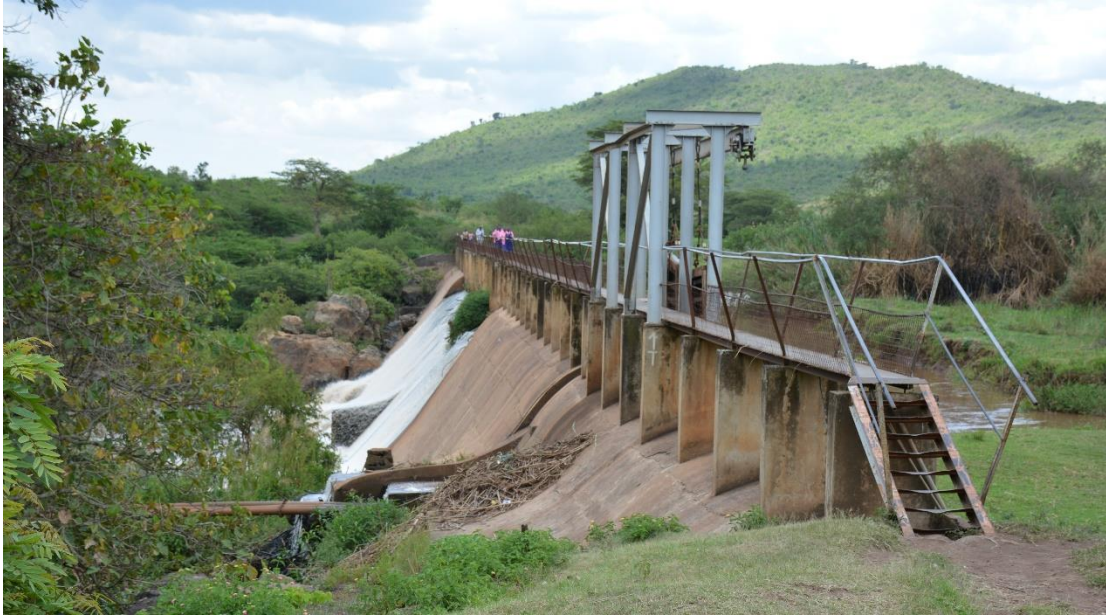
The 2MW Gogo Falls hydropower dam in Uriri sub-county still uses the generators installed in 1957. It was built to supply power to the local gold mine, but now feeds into the national grid. Photo by Oliver Johnson.
