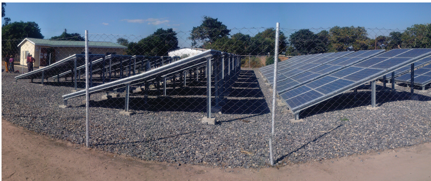
Working with development partners, Zambia built a 60 kW solar PV mini-grid in Mpanta, providing power to a rural area not served by the national grid.
