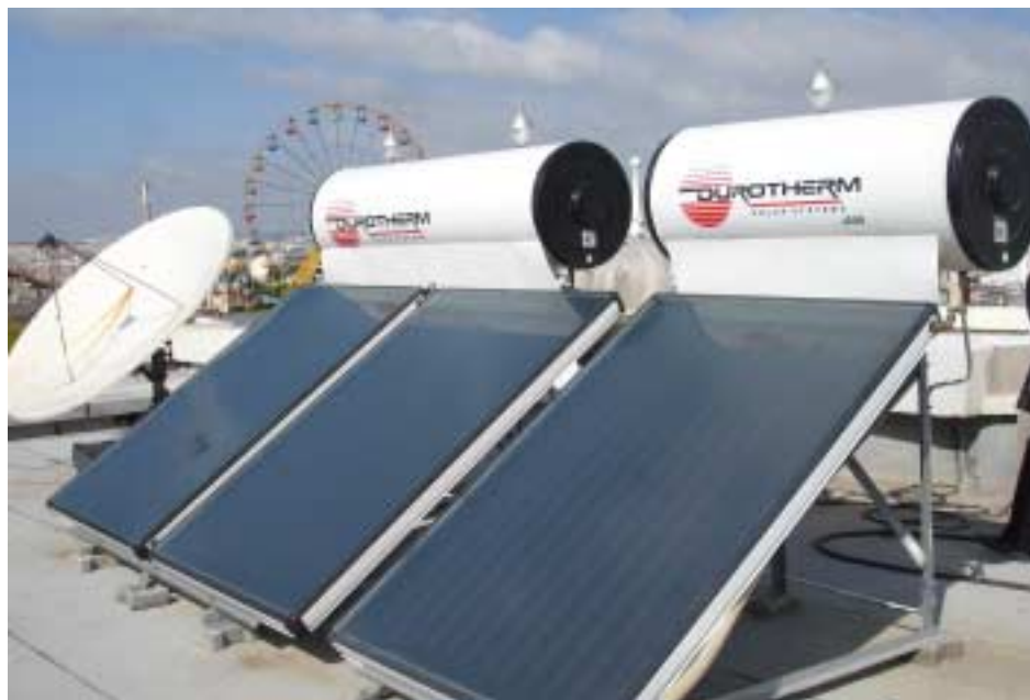
Solar thermal installation, Tunisia
