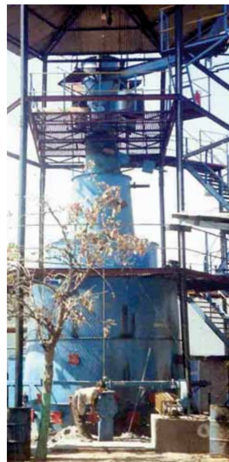
Medium-scale gasification plant, GP Green Energy Systems Pvt Ltd.
