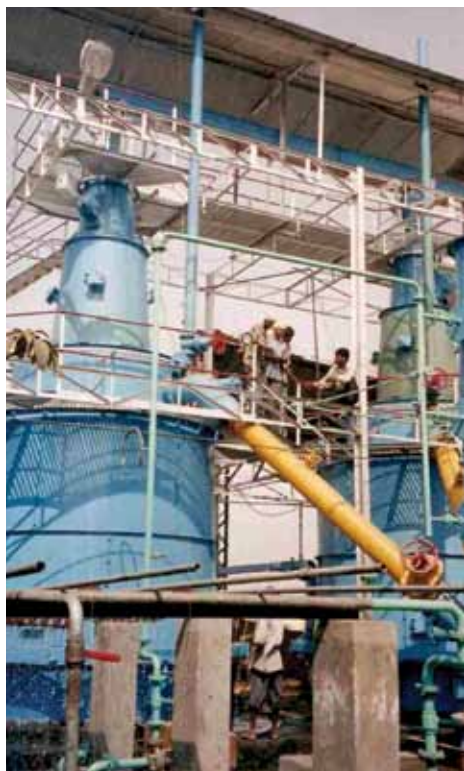
Medium-scale gasification plant, GP Green Energy Systems Pvt Ltd.
